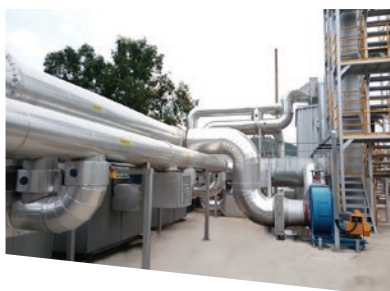
惠陽塗料廠房的VOC處理設施 Huiyang coatings plant's VOC treatment facility
