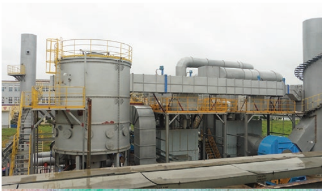
上海塗料廠房大型VOC處理裝置已全面運作。 The large VOC treatment devices in Shanghai coatings plant are fully operational.
