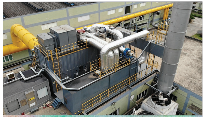
中山塗料廠房的VOC處理裝置現正進行試運行。 The VOC treatment devices in Zhongshan inks plant are now being trialed.
