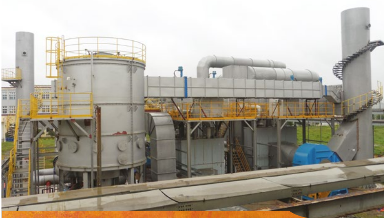
VOC處理裝置 VOC treatment device
